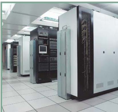
Data centre cooling
